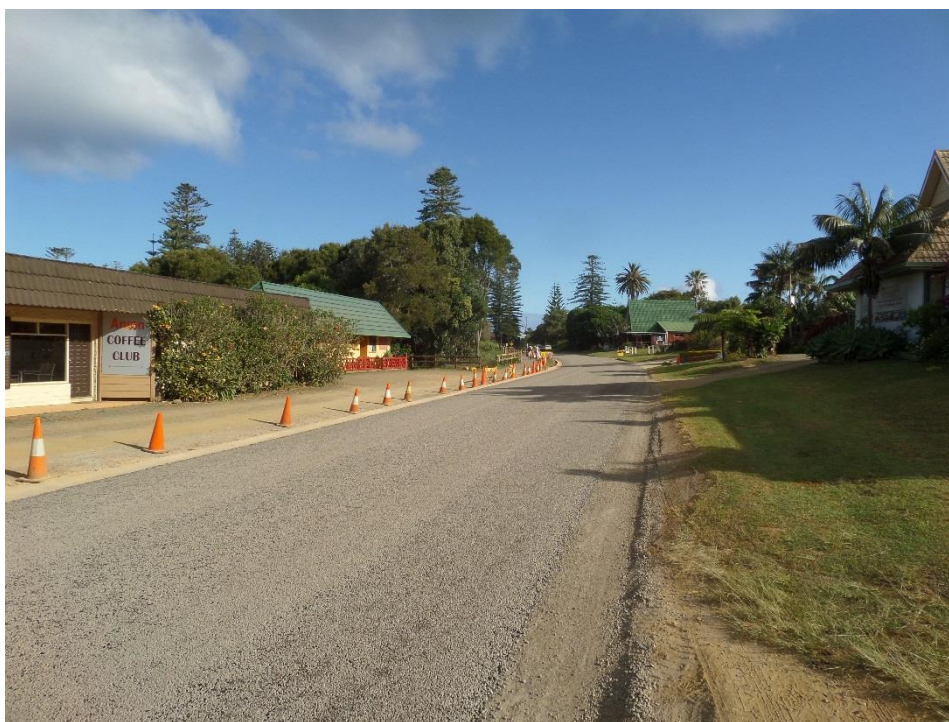
Photo shows the completed road works when the road was first re-opened again on Thursday, 20 October 2016
